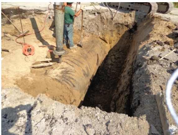
Venting the Tank
